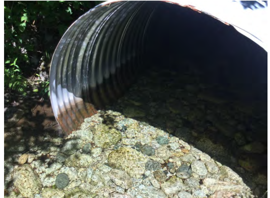
Typical Coating Condition
